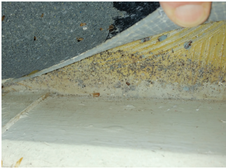
COCKROACH HARBOURAGE UNDER FLOOR LINO
