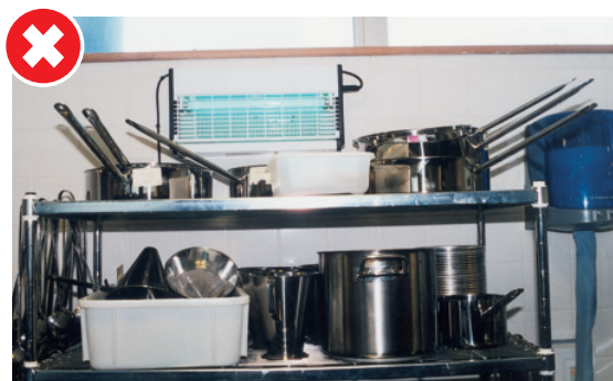
Electronic fly killer exposing clean food containers to risk of contamination
