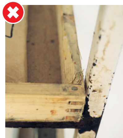
Hazards from wood splinters, rust and flaking paint
