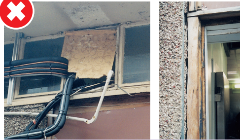
Poor maintenance will allow pest entry
